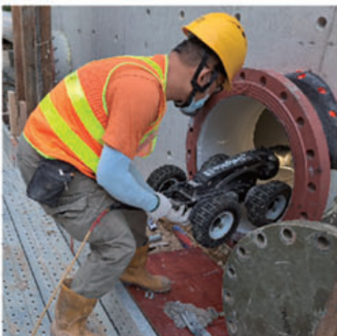
透過閉路電視勘测水喉狀況 Checking Condition of Watermain by Closed Circuit Television Survey
