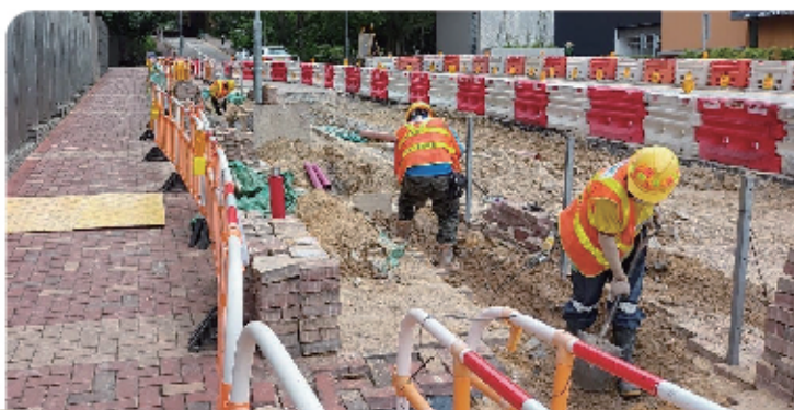
於青盈街進行鋪設公用管道挖掘工程 Trench excavation for laying utility works on Tsing Yung Street
