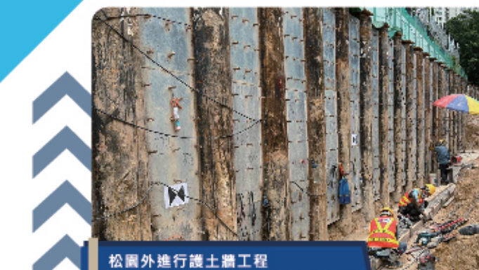
松園外進行護土牆工程 Construction of Retaining Wall outside Pine Villas
