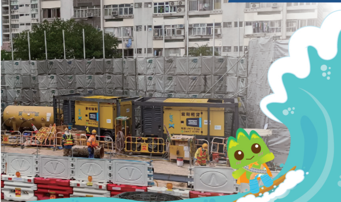
於三聖邨加裝臨時隔音屏障 Erected Temporary Noise Barrier at Sam Shing Estate
